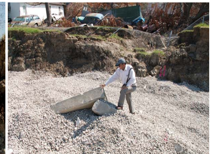
Fig. 4: Professor Sharma inspects the concrete cap panels separated from the sheet piles and moved outward.
